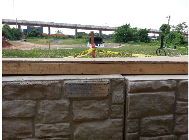
View south from north face. Contractors using block wall as work surface.
