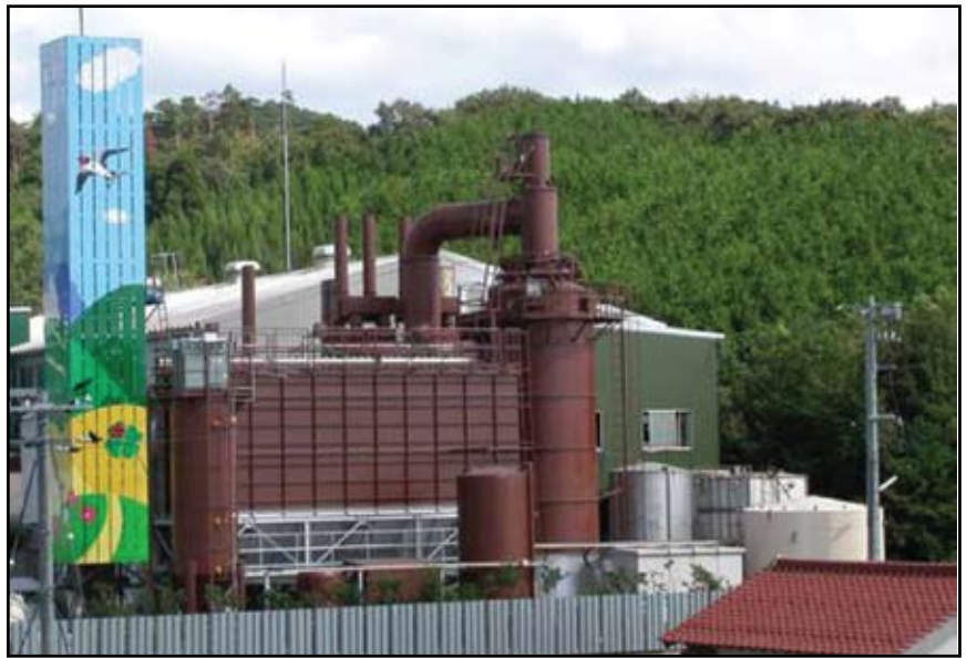
FIGURE 3. This is a general view of the filter plant and direct cooling chamber at Honshu I. The ceramic filter plant can be seen center left in the plant. To the right of the filter plant is the direct cooling chamber and to the left the exhaust stack
