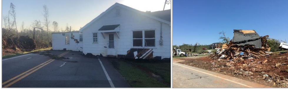
Left: In Upson county, an EF-3 tornado lifted a house from its foundation and dropped it in the middle of a road (source: WSB-TV). Right: Another house destroyed by the same tornado (source: NWS).
