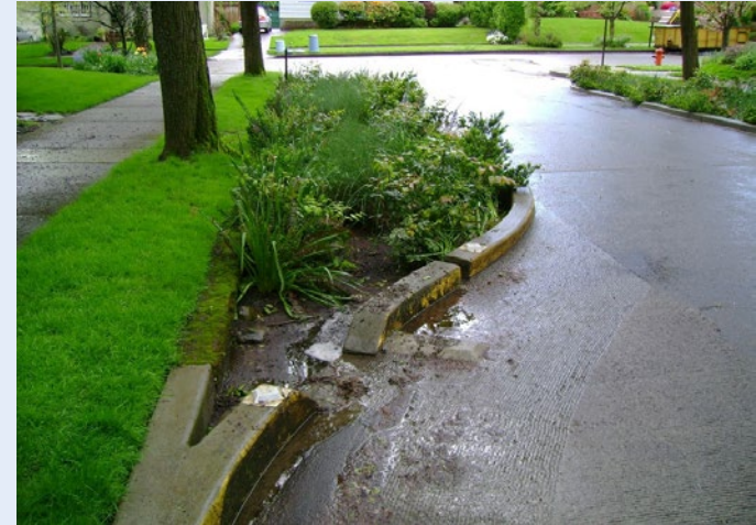
An early curb extension inlet design allowed flow bypass.
