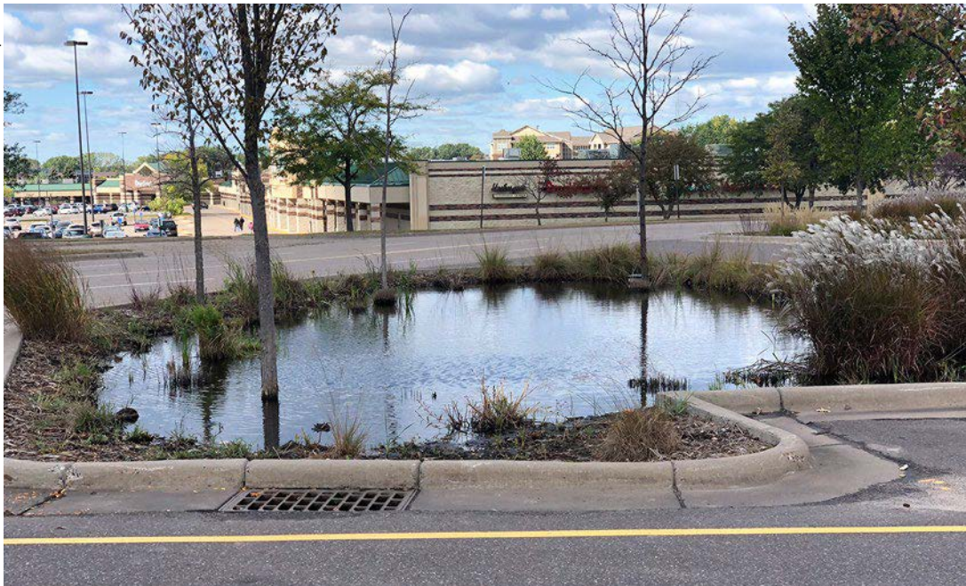
Ponded water remained for days after a storm, indicating poor drainage due to soils or outflow design.
