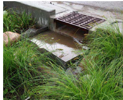
Curb Well Forebay (City of Omaha)
