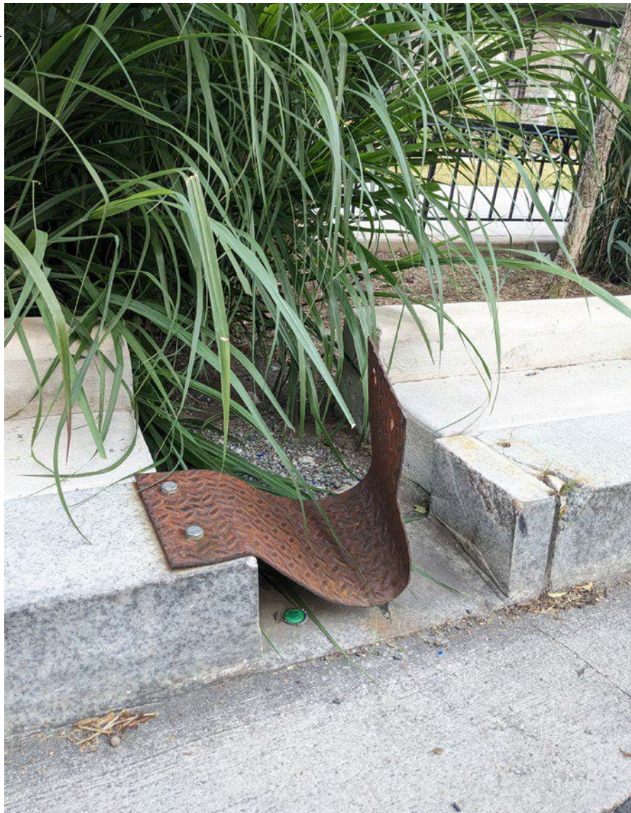
A damaged wheel guard over a curb cut in Washington, DC.
