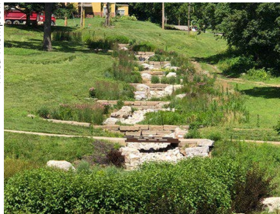
Rock check dams on a steep facility in Kansas City, MO.
