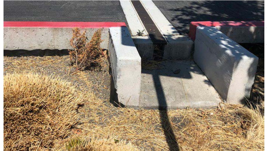
Concrete splash pad in San Mateo, CA
