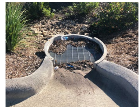
Inlet Sump Forebay (Rhea Thompson)
