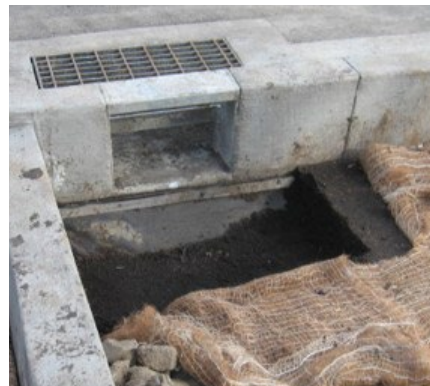
Depressed Drain (Portland Bureau of Environmental Services)
