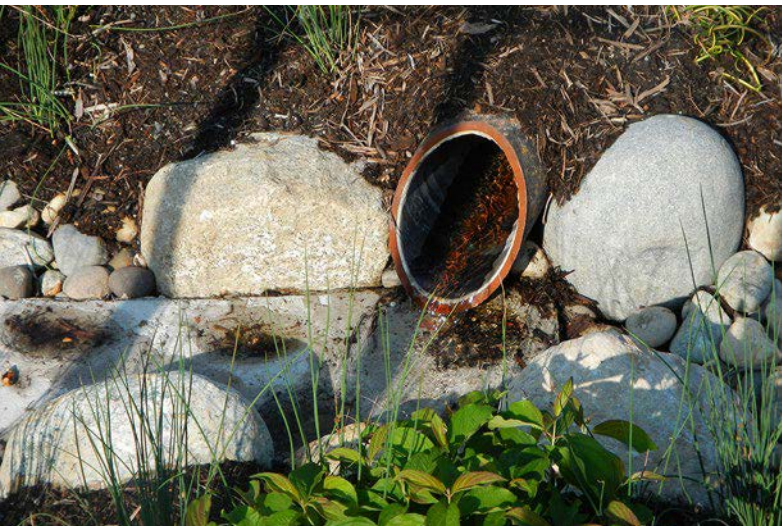
A pipe discharges runoff over an energy-reducing concrete splash pad in Seattle, WA.
