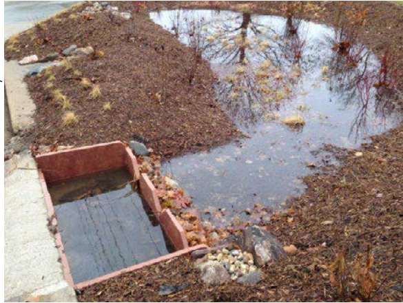
A flagstone forebay in Omaha, NE.
