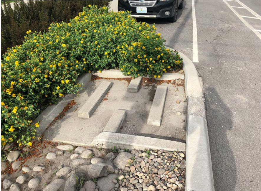
A concrete splash pad is paired with a stone forebay in Kansas City, MO.
