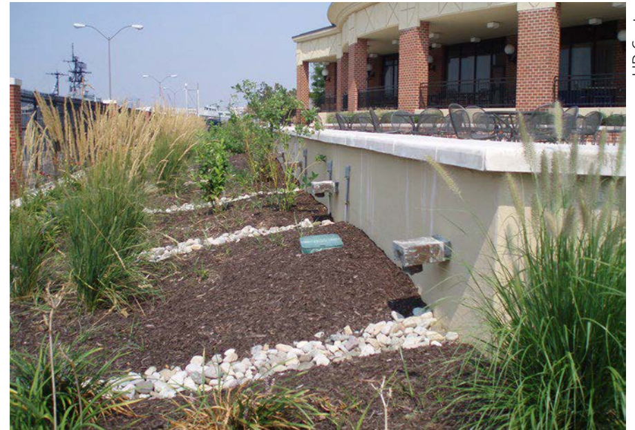
An infiltration planter treats runoff while adding aesthetic value to an outdoor space at the Navy Yard in Washington, DC.
