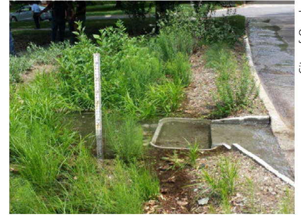
A utility box forebay in Omaha, NE.
