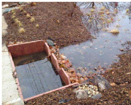
Flagstone Forebay (City of Omaha)
