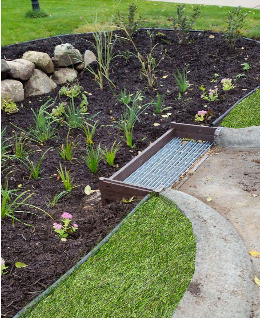
A bioretention practice in Minneapolis, MN, with a proprietary inlet sump often used in residential areas.
