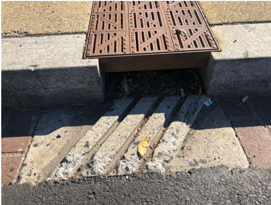
Saw cuts help direct water flow into an inlet.
