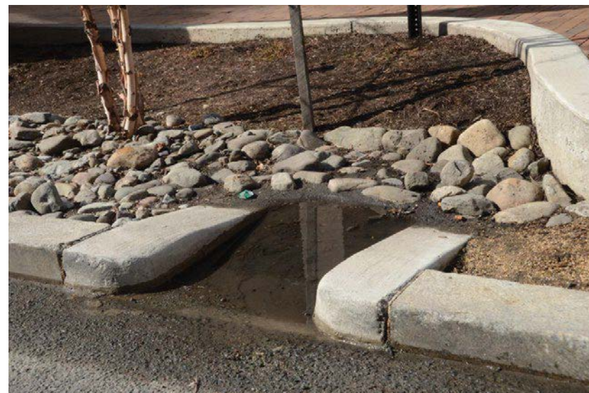
Incorrectly installed inlet.
