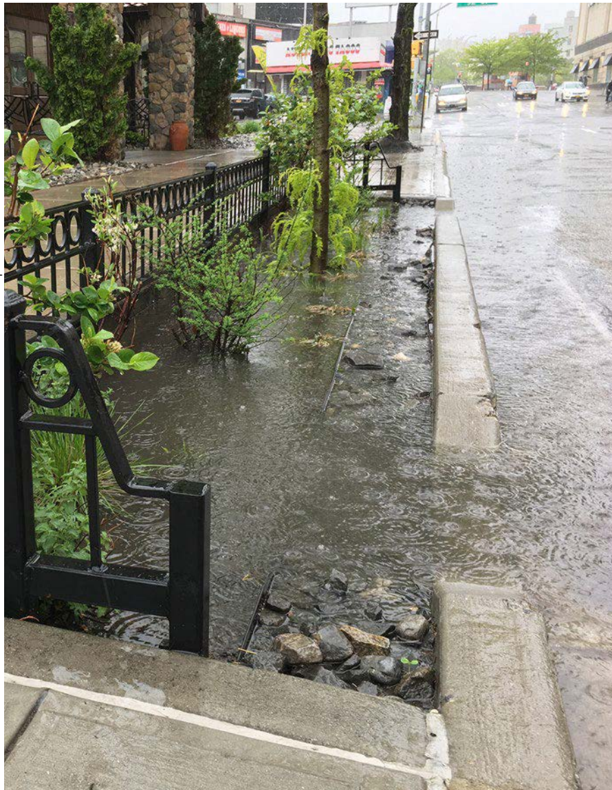
Flow enters a well-designed curb cut in New York City, NY.
