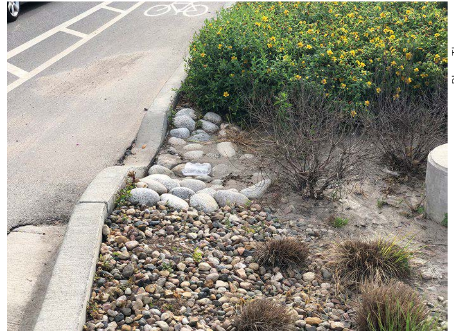
A sediment-clogged stone forebay.
