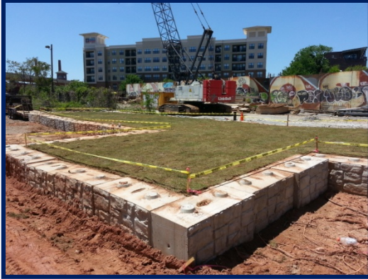
View looking southwest of final soil-vegetative cap on the NW corner of 670 DeKalb Avenue.
