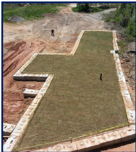
Southerly view from Edgewood Avenue Bridge of the final soil-vegetative cap on the NW corner of 670 DeKalb Avenue.
