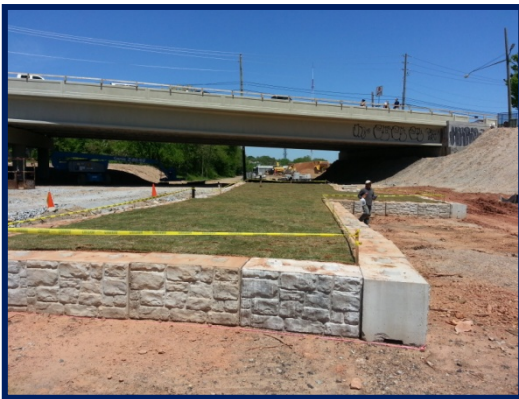
View looking north of final soil-vegetative cap on the NW corner of 670 DeKalb Avenue.
