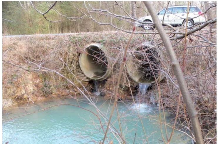
Figure 3.4. Overshot, failed culvert on E. Hermitage Road. Note the milky appearance of the water.
