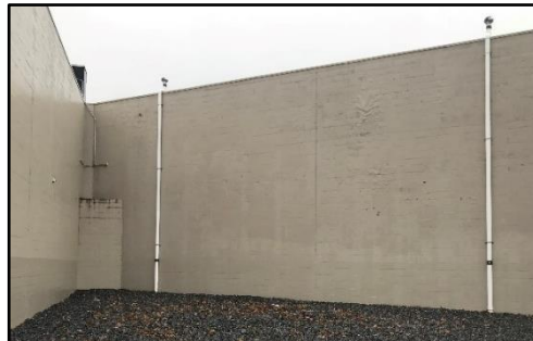
Vapor intrusion remediation system installation, Fulton County
