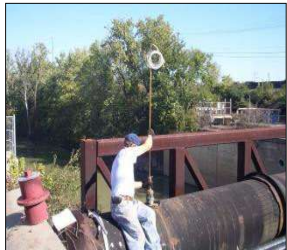
Figure 3 Pitot rod inserted into large pipeline
