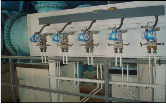
Fig 6 Bank of Differential Pressure Cells connected to flowmeters
