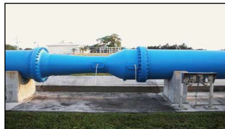
Figure 6.4 - 36-inch Venturi Meter
