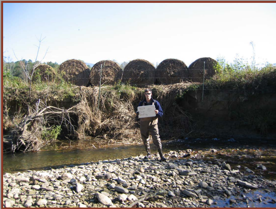
Figure 3.2.c. The above photo is a picture from the Google Earth interactive map documenting a lack of riparian buffer and a vertical, continuously eroding streambank along Holly Creek. Vertical, earthen streambanks tend to slough off massive amounts of sediment into streams making life difficult for sensitive aquatic organisms downstream.
