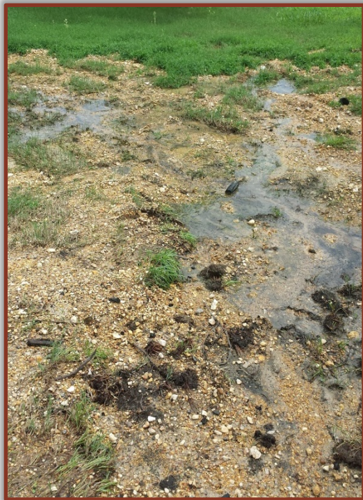
Figure 4.1.g. A failing septic system can introduce pathogens into nearby streams. This system has effluent surfacing in the yard, and drains into a nearby tributary.
