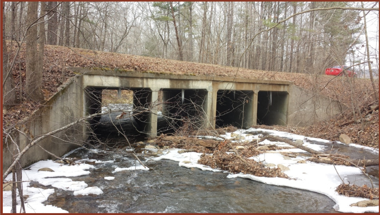
Figure 3.3.c. A photograph of the box culvert that spans Mill Creek on Holly Creek-Cool Springs Road. The structure is the least ideal along Mill Creek, but does appear likely to allow fish passage during most hydrological conditions.
