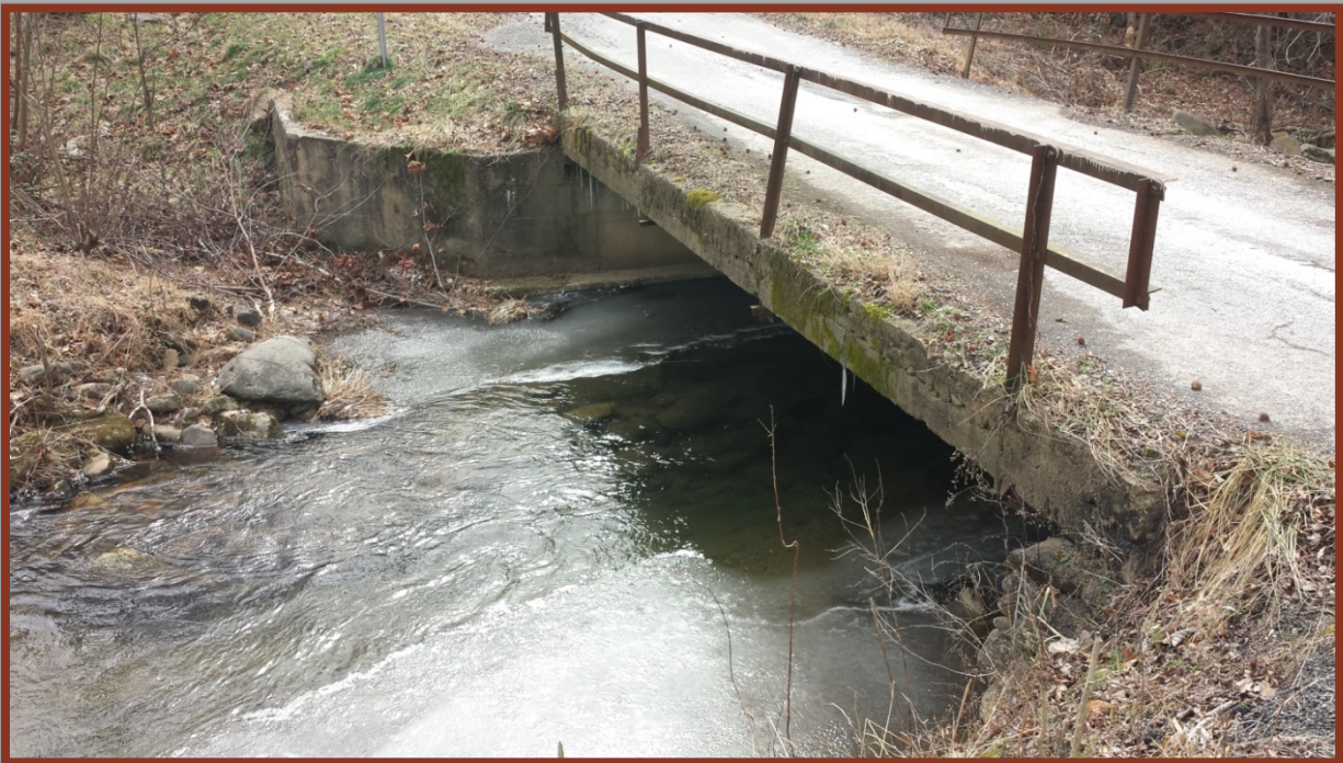
Figure 3.3.d. The free span bridge that spans Mill Creek on Hassler's Mill Road.
