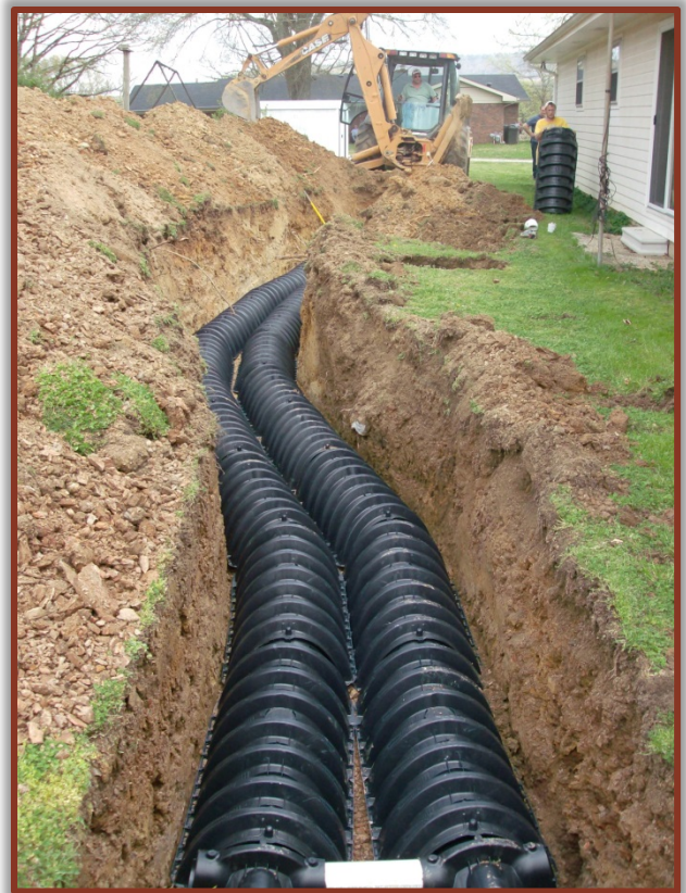
Figure 6.2.b. A septic system repair can reduce the fecal coliform load in streams. A cost-share program can help incentivize costly repairs.
