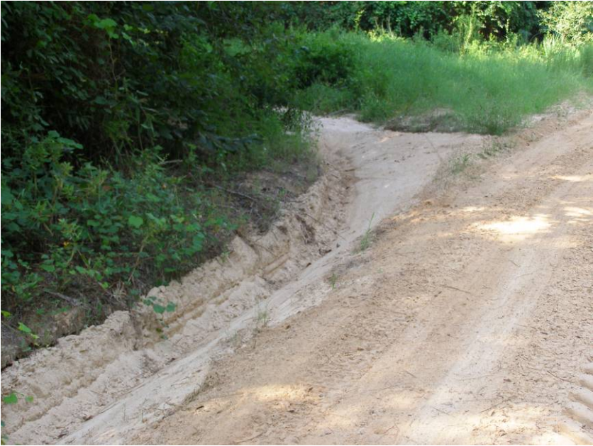
An example of a water turnout at the bottom of the hill that directs the water into the stream.
