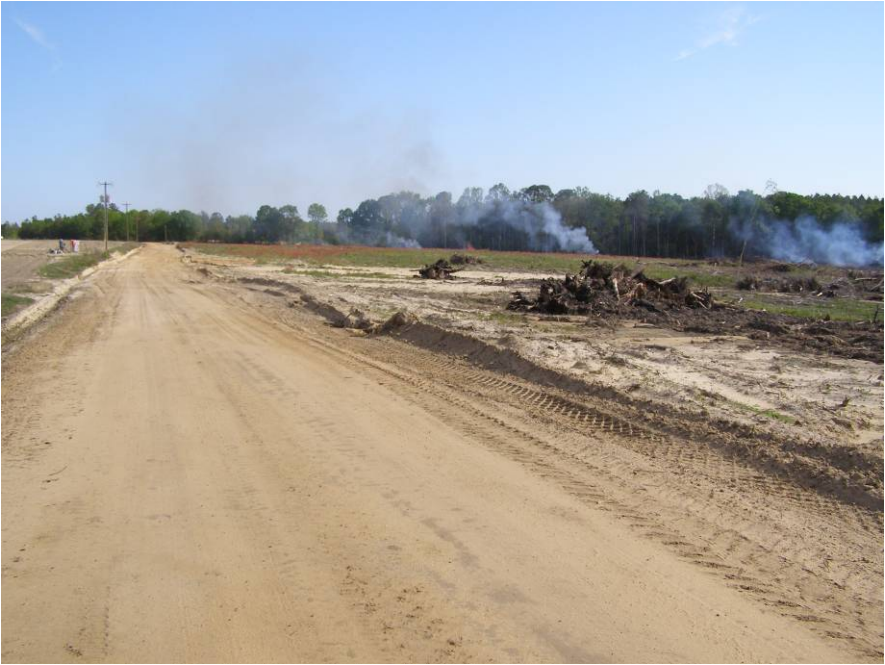
The county road is receiving sediment from an adjacent land clearing operation. The landowner and county are working to resolve the problem.
