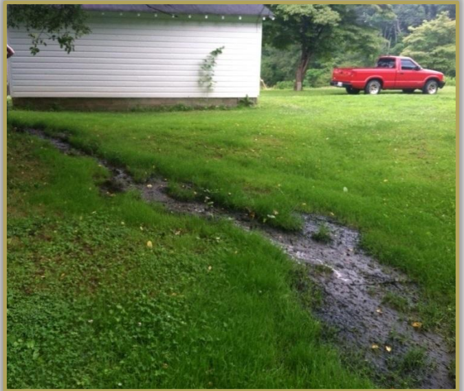
Figure 4.1.c. A failing septic system can introduce pathogens into nearby streams. This system has effluent surfacing in the yard, the vast majority of which drains into a nearby tributary.
