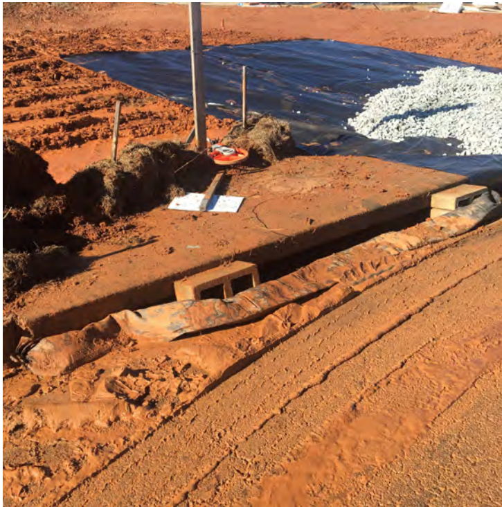
Inadequate compliance with Erosion and Sedimentation ordinance.
