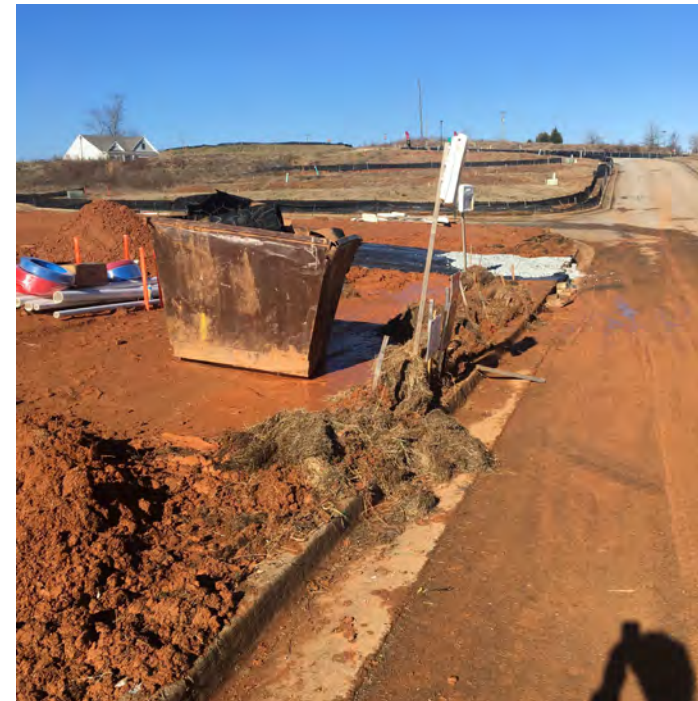
Inadequate compliance with Erosion and Sedimentation ordinance.
