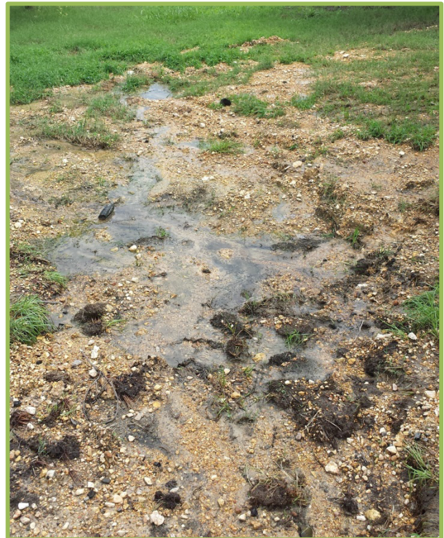
Figure 5.1.a. Effluent surfacing from a failing septic system.
