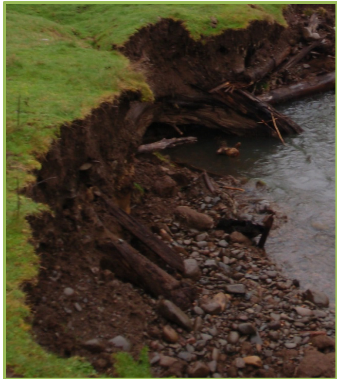
Figure 6.2.a. Eroding streambanks contribute to sediment loads in the watershed.
