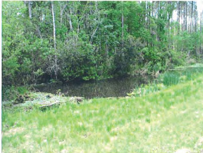
Ponding by Beaver Dam Southside of St. Marys Scrubby Bluff Sewage Plant Access Road
