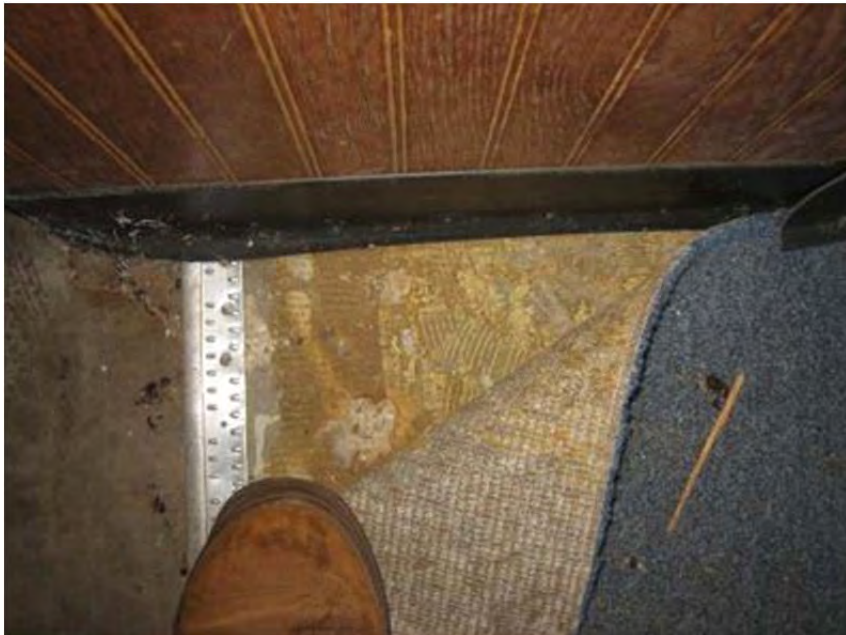
Photo 7: Non-ACM yellow carpet mastic in dry cleaners.
