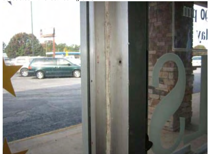
Photo 12: Non-ACM white caulk around entry door of nail salon.
