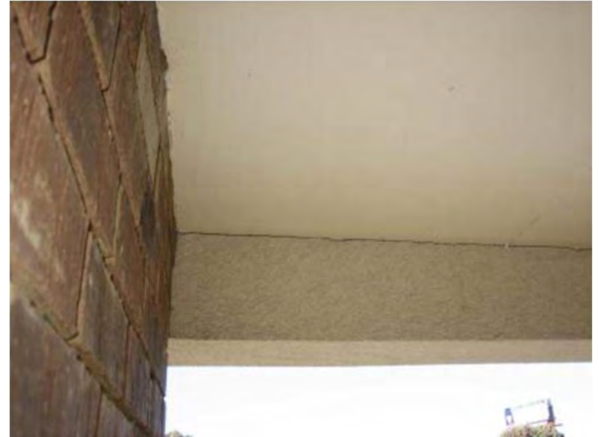
Photo 14: Non-ACM EIFS and wood overhang of strip center.
