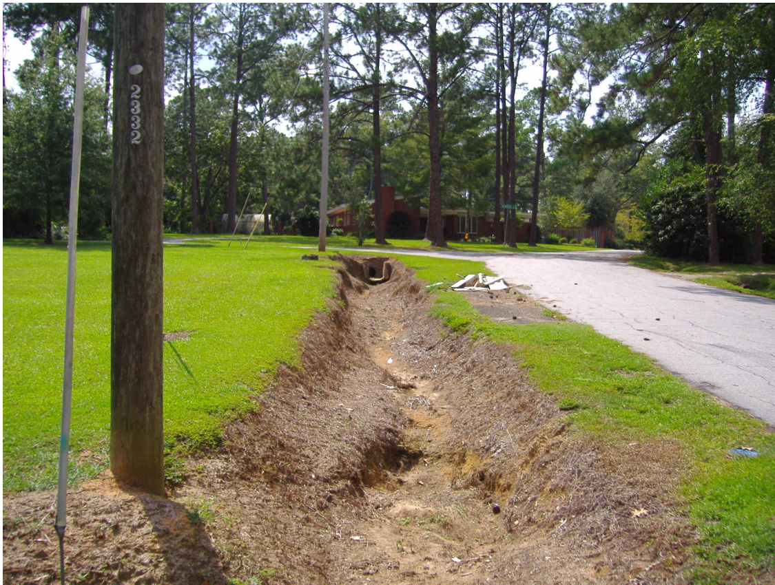
Figure 12. Eroding roadside ditch
