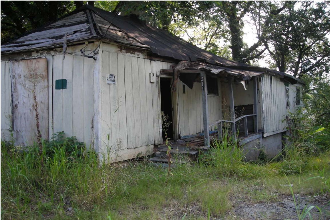
Photo No. 7: View of dilapidated house in southwest portion of the site.
