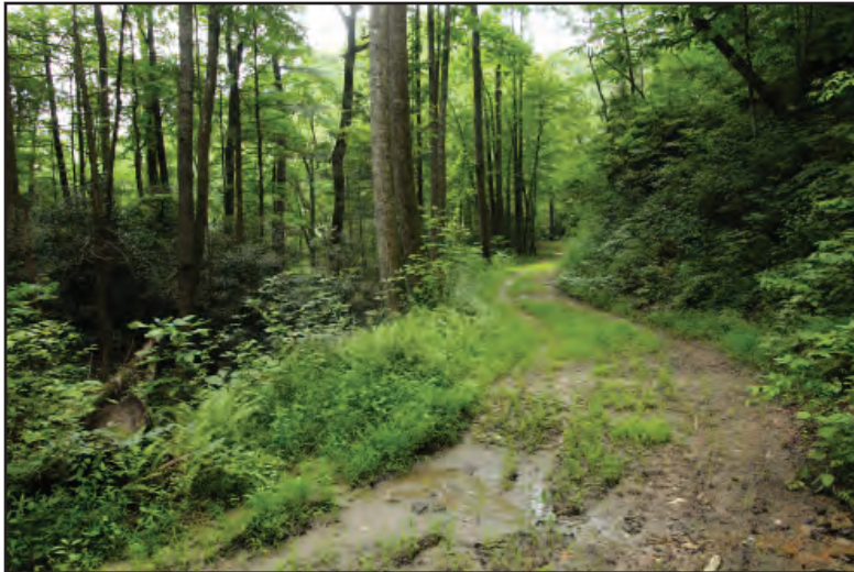
Gravel roads lacking stormwater BMPs and structural controls are a primary source of sedimentation into the Warwoman watershed.
