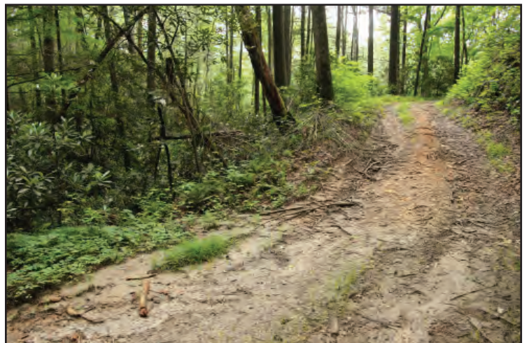
FS 155A is a large sediment source to Walnut Fork due to lack of maintenance and the road's close proximity to the stream.
