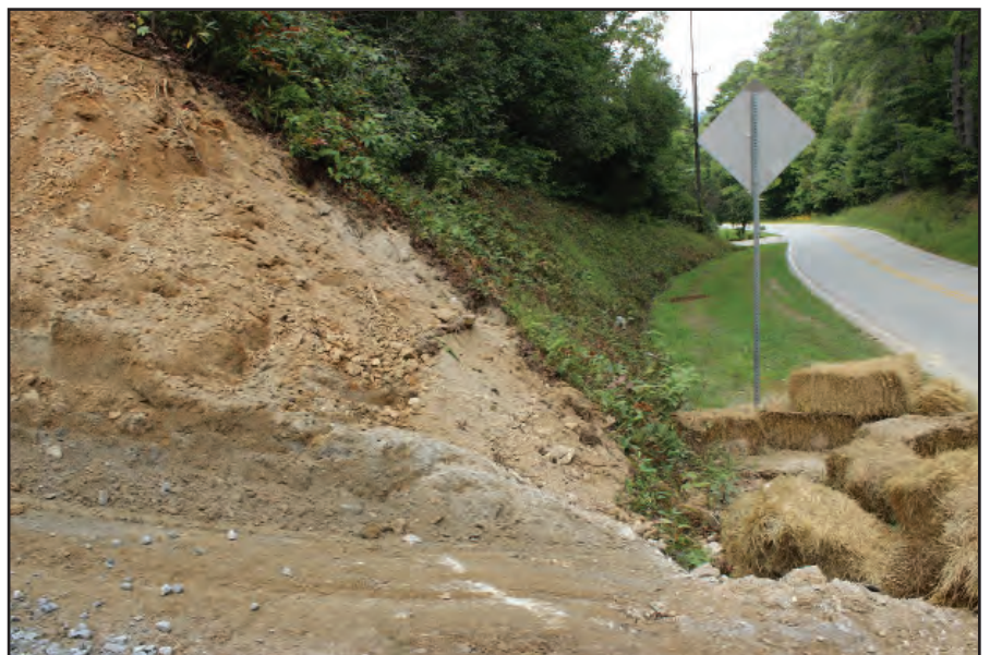
New construction on Warwoman Rd. with minimal stormwater management could create increased sedimentation into Warwoman Creek.
