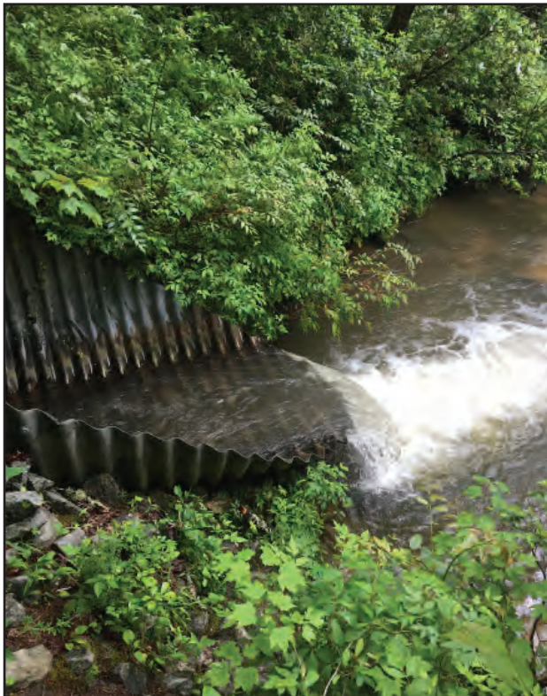
Reed Mill Creek flows through a large culvert into the West Fork of the Chattooga River.
