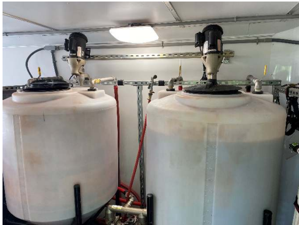
Injection Mix Tanks
