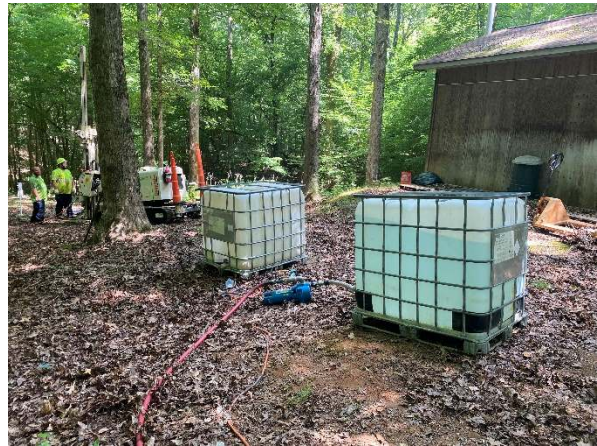
Dilution Water Transported in 250 gal Totes
