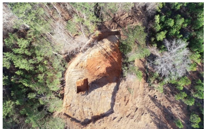
Excavation at the Former W.F. Harris & Sons Wood Preserving Site in Upson County
