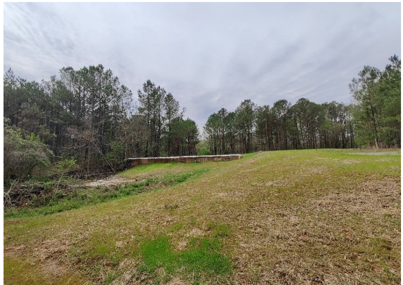
Soil cap with seed and straw at the Palmetto Tire Fire Site.
