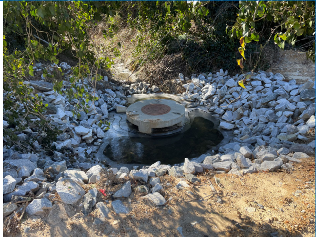
Photo 4: Surface water drop inlet
