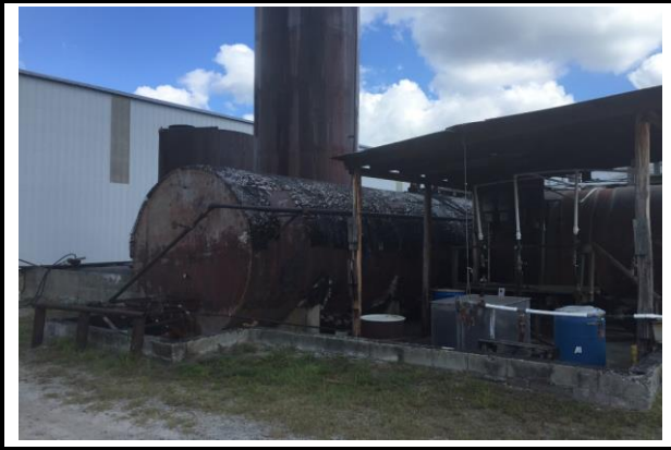
View: The activated carbon system was observed within a bermed area located in the center of the facility.
