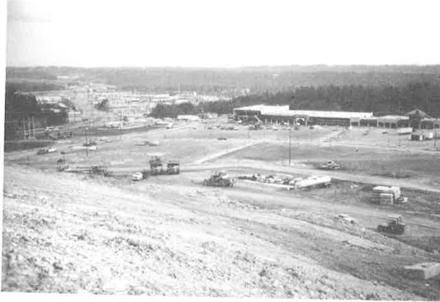
Figure 12 - View southeast down slippage plane of second block slide toward completed shops across Festival Centre terrace in January, 1989. Two buildings are planned for location at the base of this slope but are enjoined at this time.
