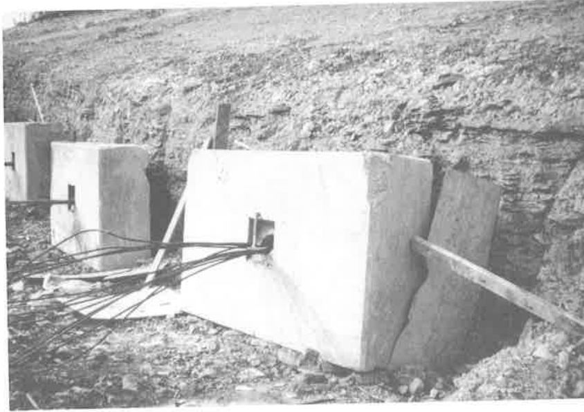
Figure 11 - Tiebacks installed at cut face in lower part of middle siltstone. Slippage plane for second block slide extends upslope from top of cut face. Cement blocks are approximately 2 feet x 5 feet x 7 feet. View looking southwest.
