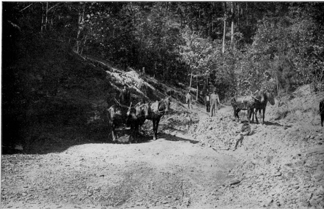
MINING FOSSIL IRON ORE BY SURFACE STRIPPING, NEAR ESTELLE, WALKER COUNTY, GEORGIA.
