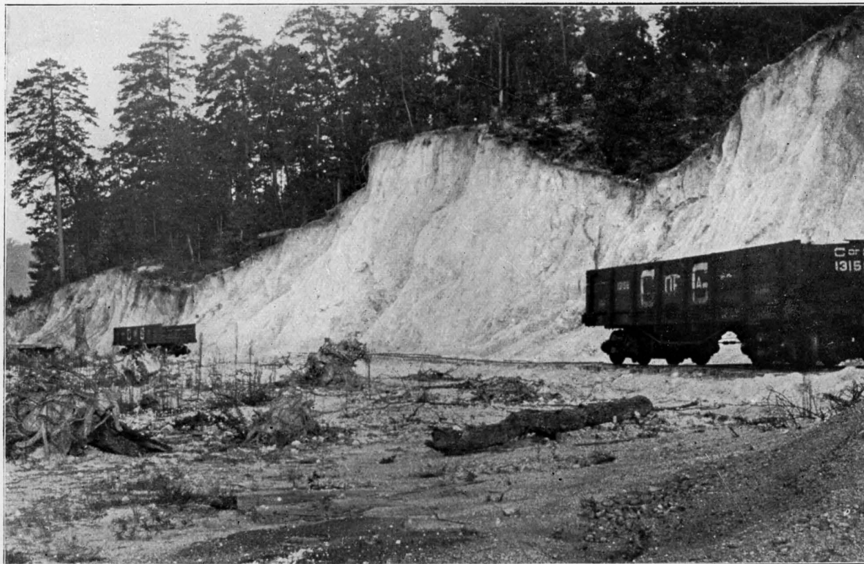
RESIDUAL CHERT AND CLAY RESULTING FROM THE WEATHERING OF THE KNOX DOLOMITE, IN A CUT ON THE CENTRAL OF GEORGIA RAILWAY, NEAR SUMMERVILLE, CHATTOOGA COUNTY, GEORGIA
