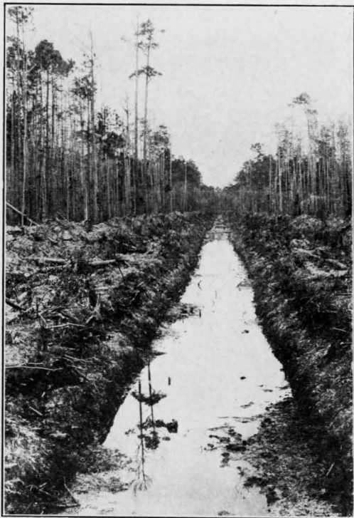
A. TYPICAL COASTAL PLAIN DRAINAGE DITCH (BUTTS COUNTY). THIS DITCH WAS CONSTRUCTED WITH A DRY-LAND DIPPER DREDGE
