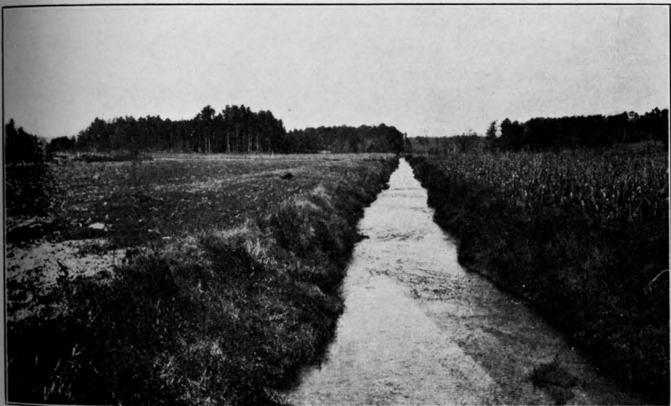
B. DITCH COMPLETED AND BOTTOMS UNDER CULTIVATION, BIG HAYNES CREEK, GWINNETT COUNTY, GEORGIA. NOTE THAT SPOIL BANKS HAVE BEEN LEVELED OFF AND LAND IS CULTIVATED UP TO THE DITCH BANKS
