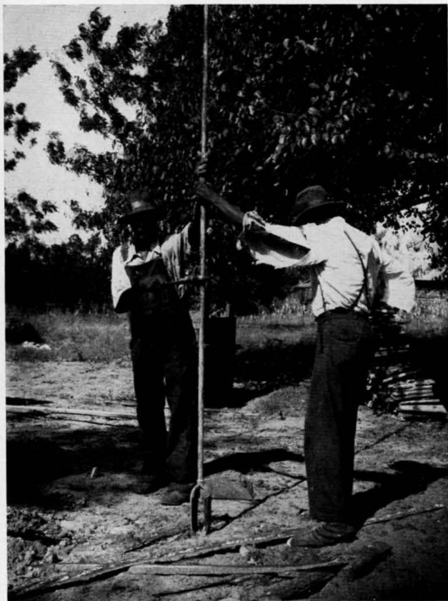
Figure 8. Simple hand auger equipment used by "Doc" Bostick, at Toombsboro, Wilkinson County, to bore shallow wells. Upon penetrating a water sand a well point is driven into the aquifer, and water is recovered by a hand pump.
