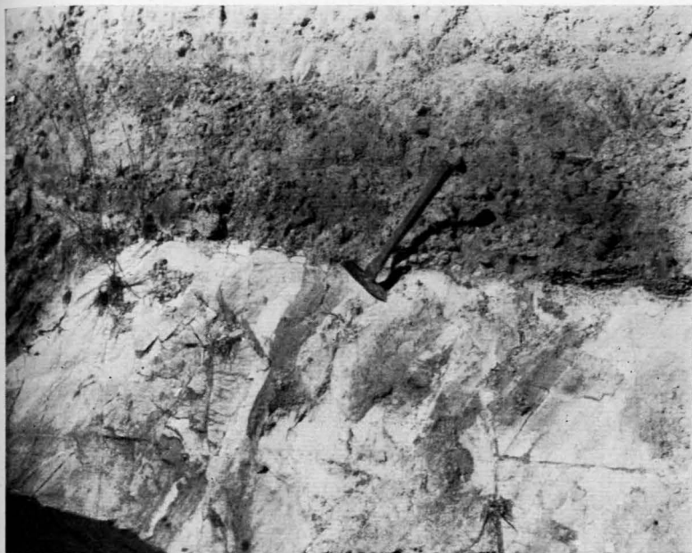
Figure 11. Road cut in Stevens Pottery-Milledgeville Road 1.8 miles northeast of Coopers School (Baldwin County) showing sand and gravel of the Tuscaloosa formation lying unconformably on deeply weathered micaceous schist of pre-Cretaceous age.
