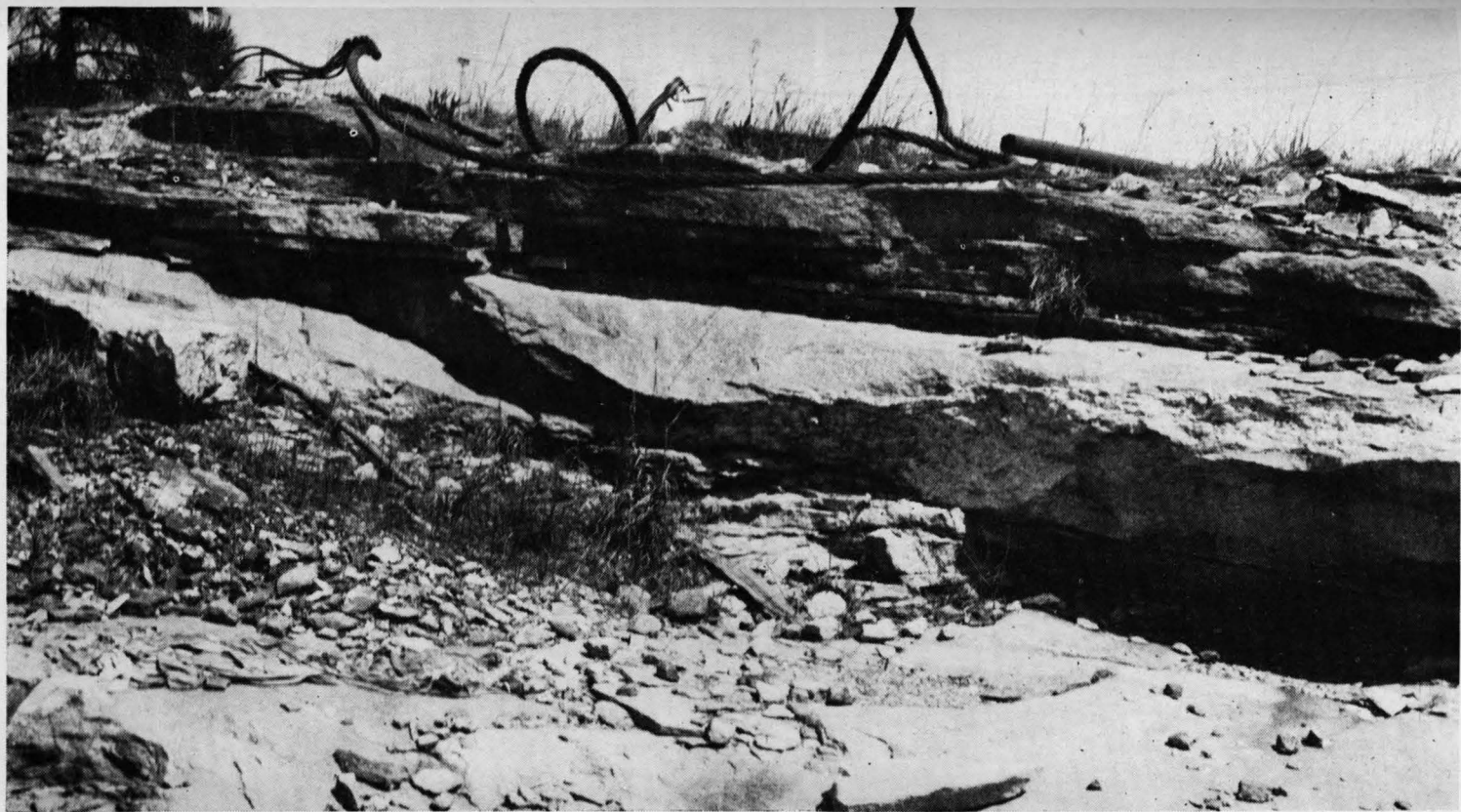
Figure 9. Exfoliation in granite at Stone Mountain quarry, DeKalb County, Georgia.
