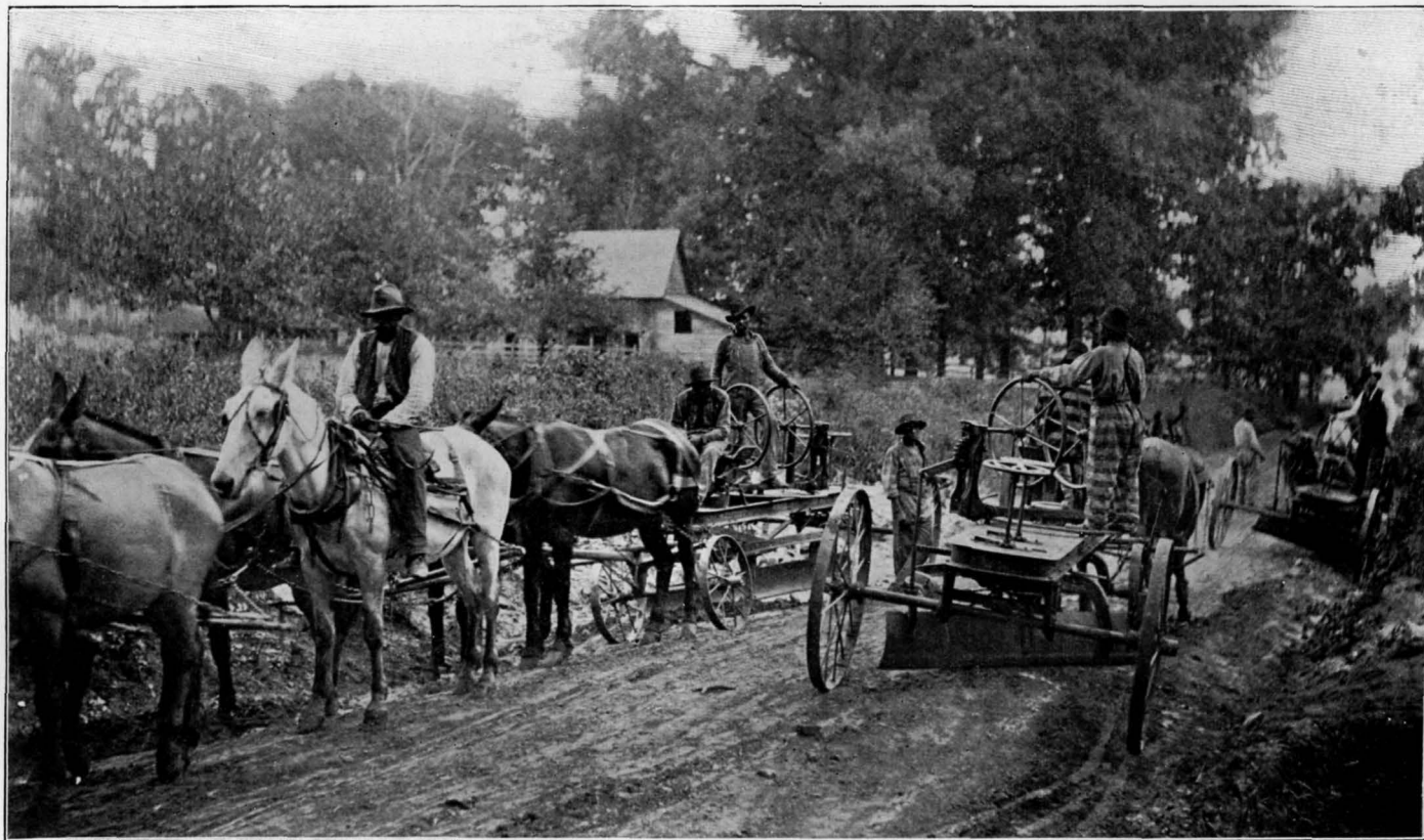
AT WORK ON THE ROAD BETWEEN DECATUR AND CONYERS, GEORGIA, SHOWING 3 OF THE ROAD-MACHINES OWNED BY DEKALB COUNTY.
