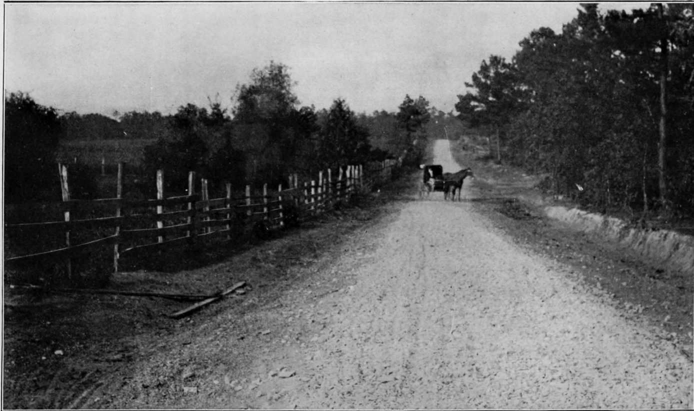
A VIEW ON THE KINGSTON ROAD, FLOYD COUNTY, GEORGIA, 3\frac{1}{2} MILES FROM ROME, SHOWING MACADAM RECENTLY PUT DOWN.
