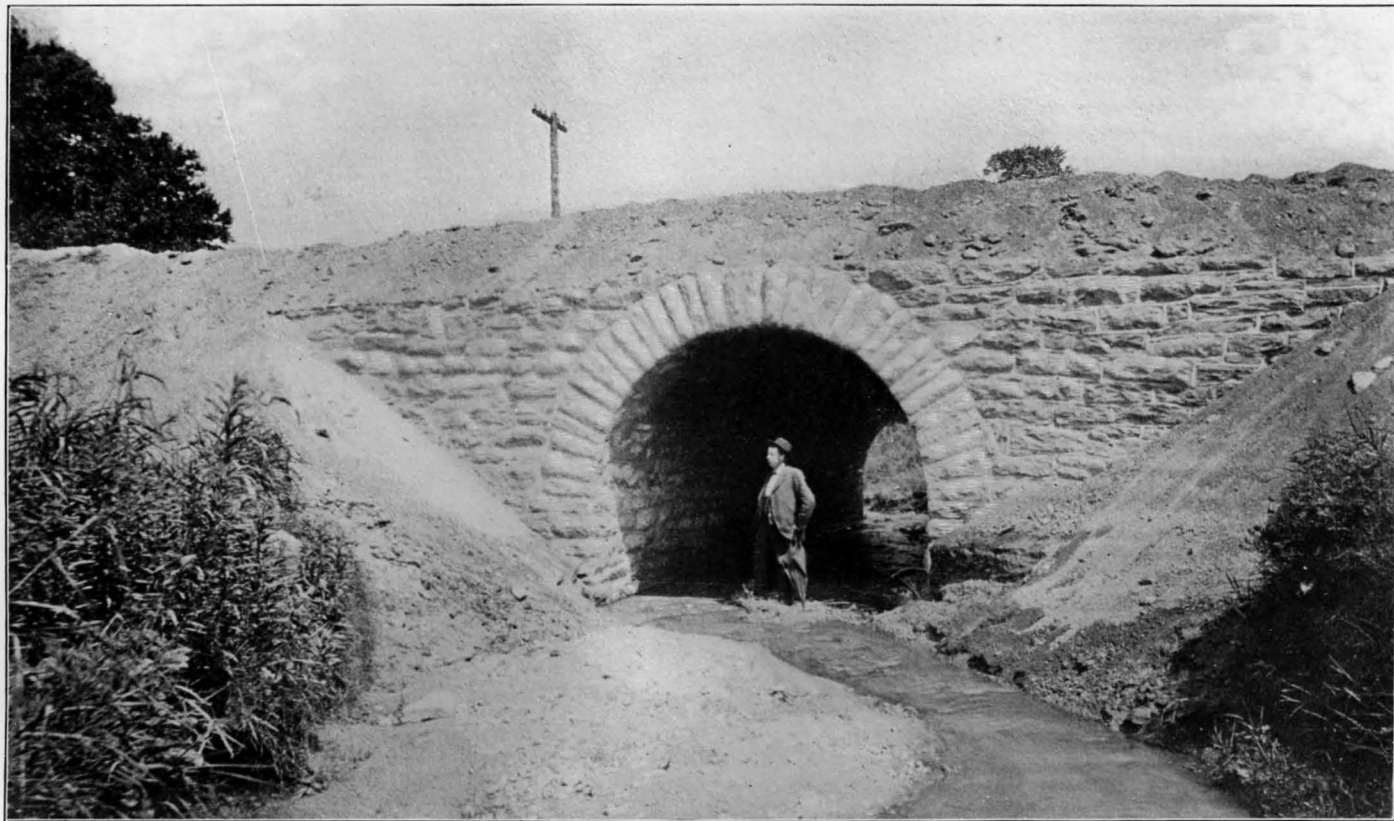
CULVERT ON BATTLE HILL AVENUE IN FULTON COUNTY, NEAR THE CITY LIMITS OF ATLANTA.
