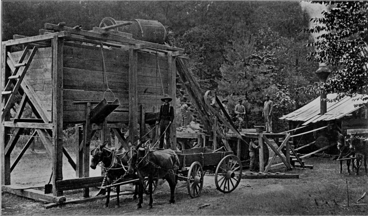
A PORTABLE ROCK-CRUSHING PLANT ON THE PEACHTREE ROAD, NEAR ATLANTA—A PART OF THE ROAD EQUIPMENT OF FULTON COUNTY.
