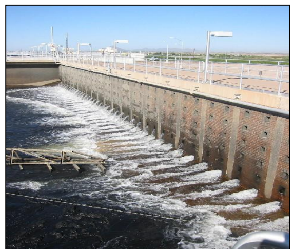
Figure 9 Reservoir or clearwell adjacent to a water treatment plant
