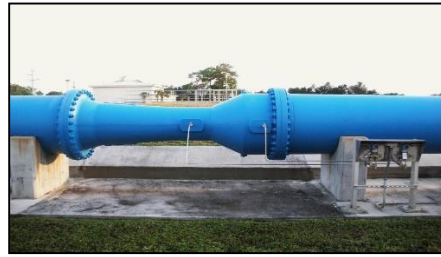
Figure 2 - 36-inch Venturi Meter
