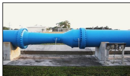
Figure 2 - 36-inch Venturi Meter
