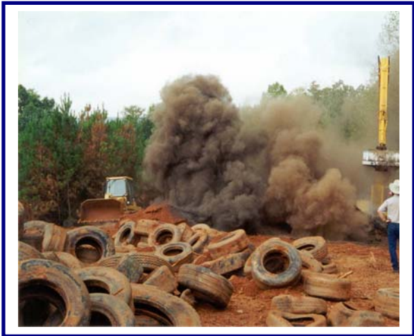
Watson Tire Fire – contractor supervising the excavation and extinguishing of burning scrap tires in the landfill.
