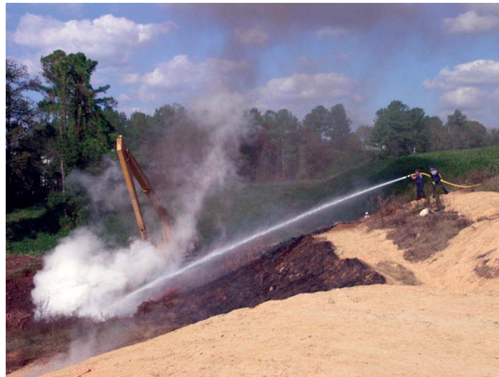
Cobb County firemen work to douse the fire at the West Sandtown Road Inert Landfill, as a backhoe mixes the burning debris with soil.
