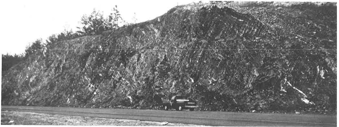
Figure 2 Type locality of the Pumpkinvine Creek Formation along Interstate 75 just south of Pumpkinvine Creek in Bartow County.
