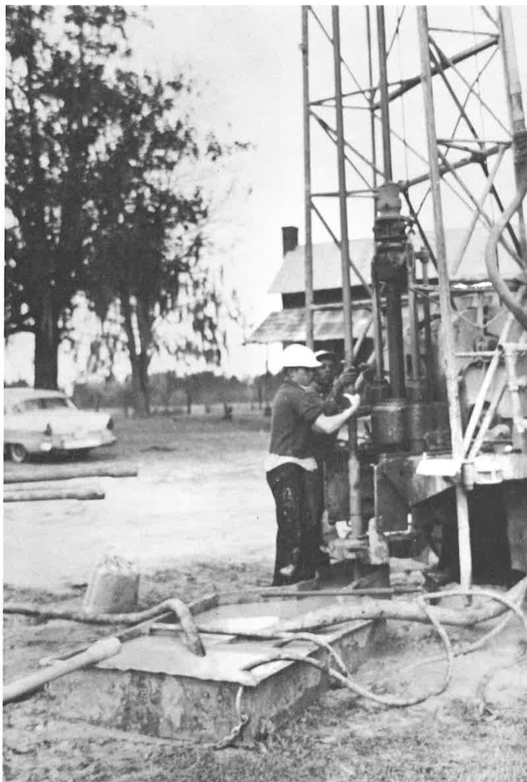
Figure 5. Disconnecting drill stem sections. Core barrel just emerging from hole. Mud pit in foreground.
