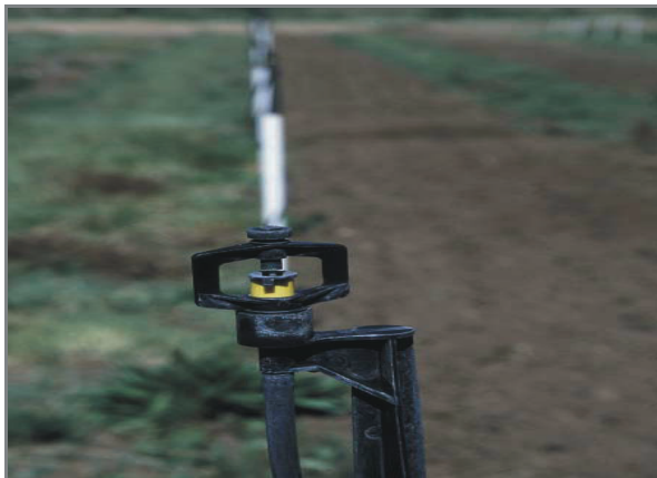
Sprinklers can efficiently apply water to targeted areas
