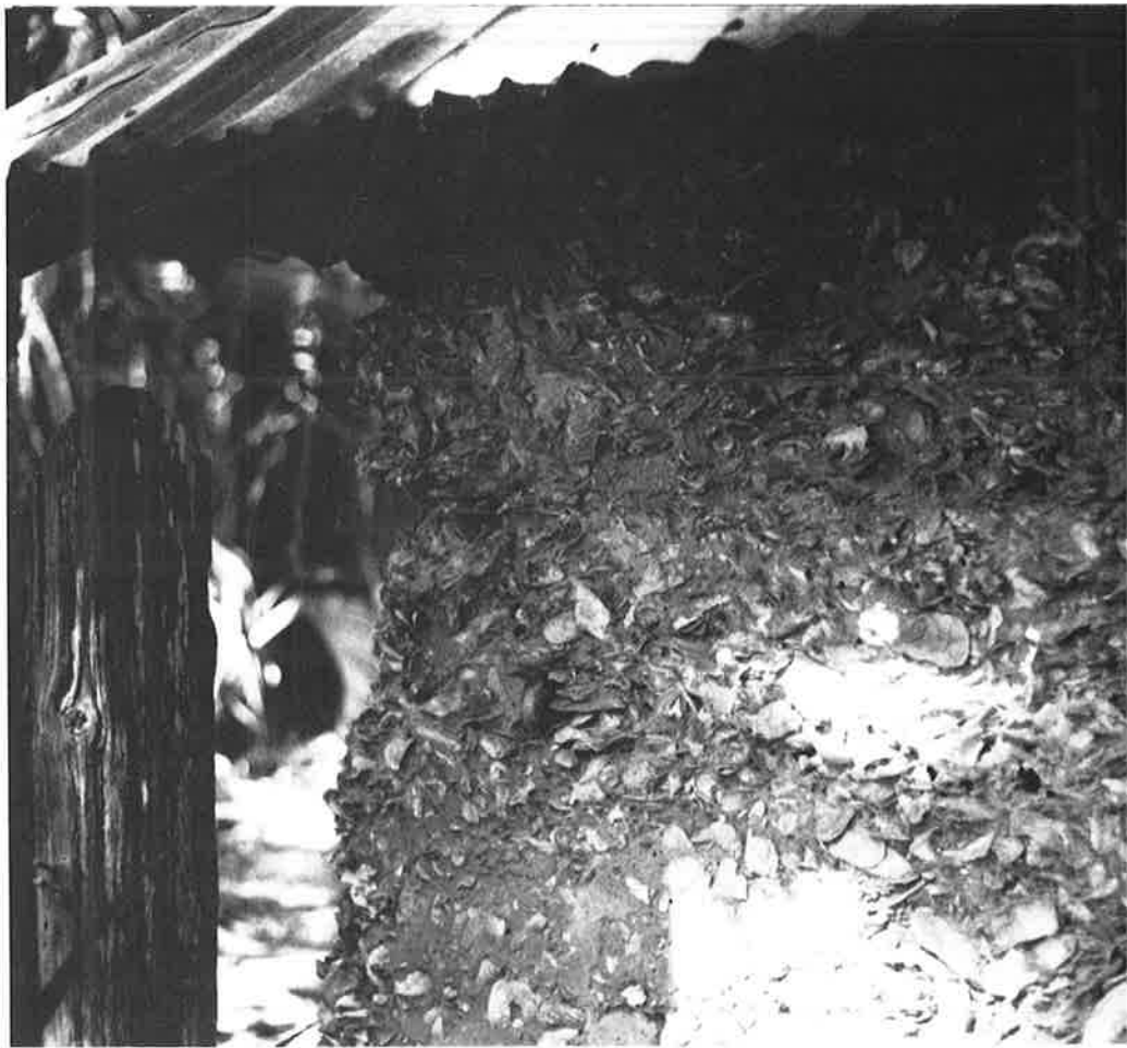
Figure 23. Tabby construction seen at the old ice house at Dungeness. The extensive use of tabby by early Cumberland Island settlers made good use of the abundant oyster shell middens.
